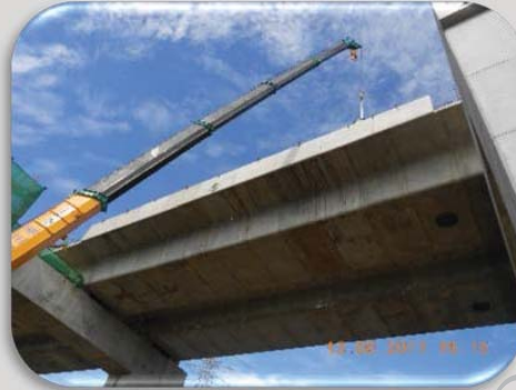
Barrier & Cable Trough
